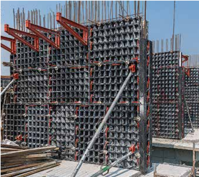
Successful first use of the lightweight universal formwork for the construction of shear walls.
