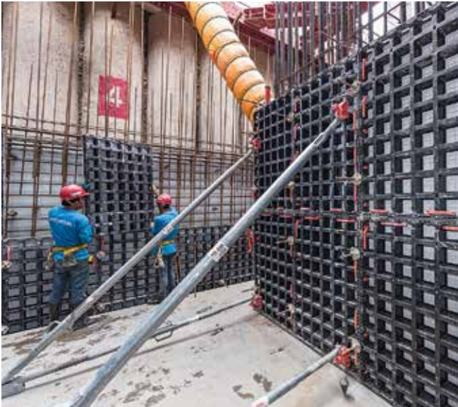
Low weight, small-format formwork elements – DUO showed off these advantages to the full with these basement walls.
