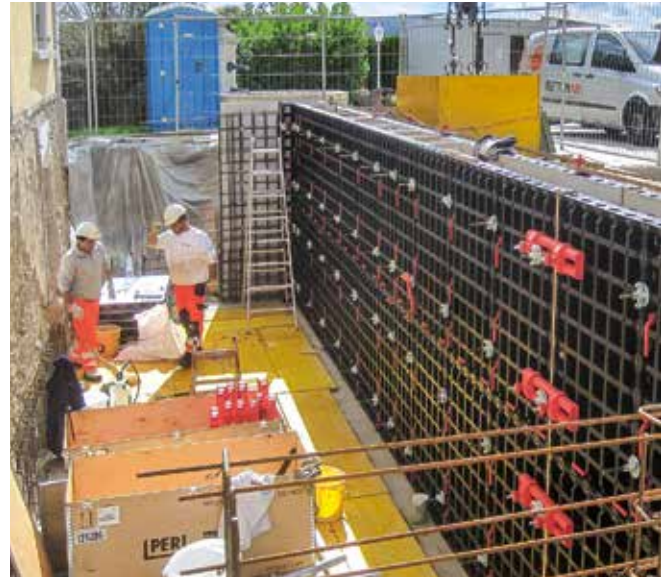
Modifications and extensions without the use of a crane - best solved with DUO.
