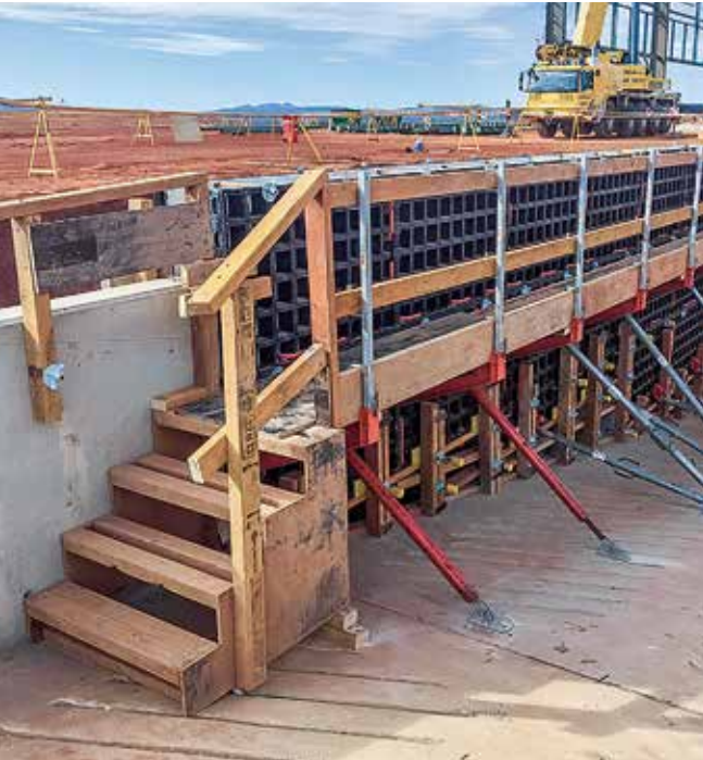
Using the DUO system resulted in a considerable increase in efficiency on the construction site.
